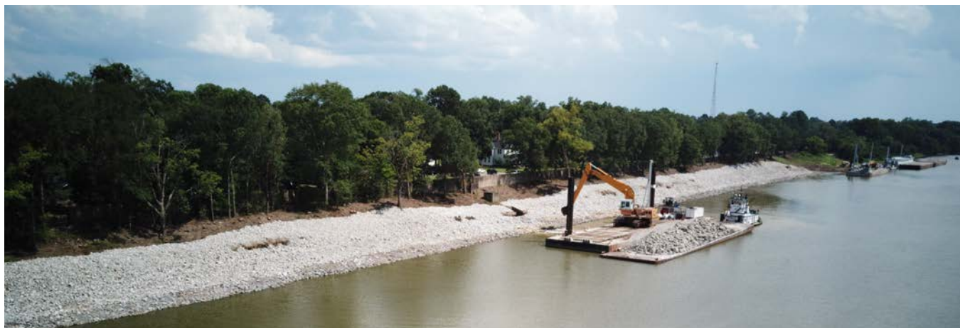
Drone photos courtesy of Jason McMillan of the Tensas Basin Levee District.
